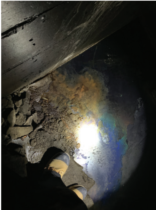
Pictured on the left: hydrocarbons pooling on the floor of the void adjacent to the subsurface concrete water tanks.
