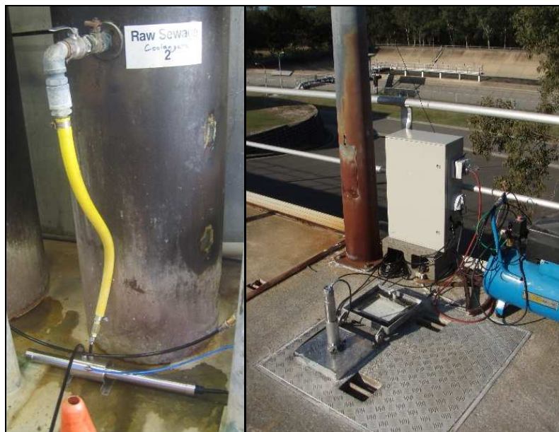
Figure 3. Deployment of the spectrometer. Site 1: in a bypass fitting and Site 3: installed in a sealed box channel.
