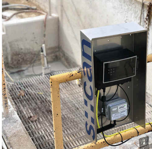
Smart sensors measure pH continuously at a permitted discharge point.
